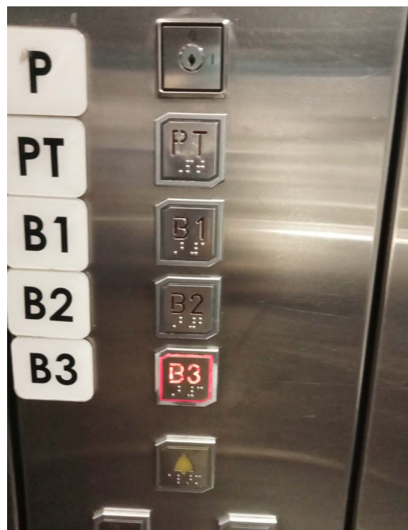
Braille and extra-large lettering on lift buttons for blind and visually impaired users.
